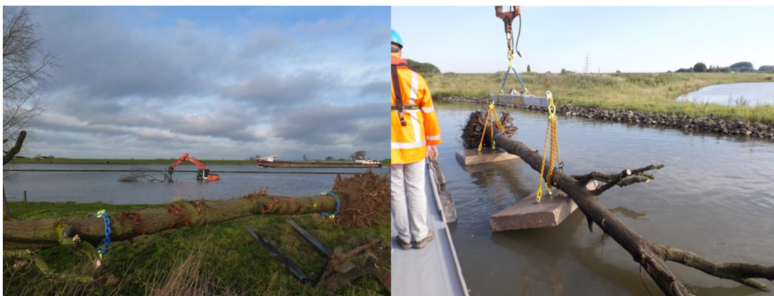
Figure 2: Entire trees were fixed in the riverbed and side channel (left) and concrete slabs were used to submerge the trees in deep erosion pits (right).
